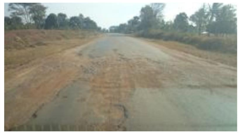
Damaged road along East-West Economic Corridor in Lao
