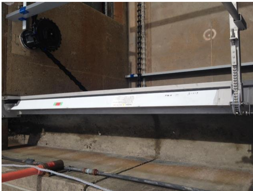
Installation in progress of Fujiwara Fuji-float scum removal system at Ashbridges Bay Wastewater Treatment Plant (Toronto, August 2015)
