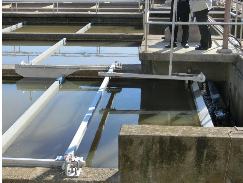
Fujiwara Fuji-float scum removal system in use at Ashbridges Bay Wastewater Treatment Plant (Toronto, August 2015)
