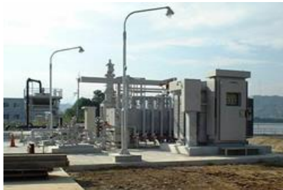
Electro Chlorination System
