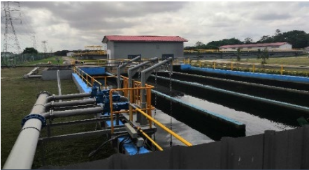
Sewage Treatment Plant ("STP")
