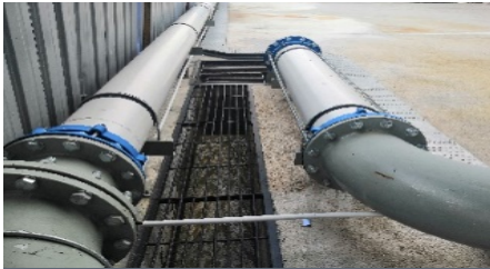
Dedicated Distribution Pipe
