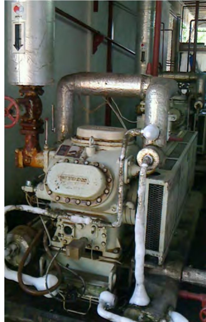
Freezing machine for refrigerator MYCOM F42WA
