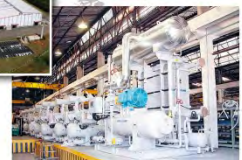
● Aruja Plant, Brazil MAYEKAWA DO BRASIL LTDA.
